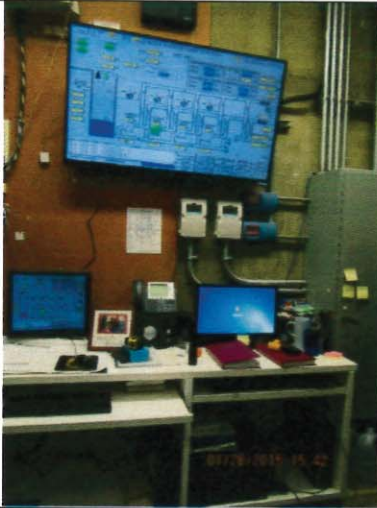
Photo 9: MAPS and SMURRF control room
