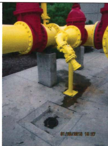
Photo 4: MAPS force main emergency bypass valve and connection
