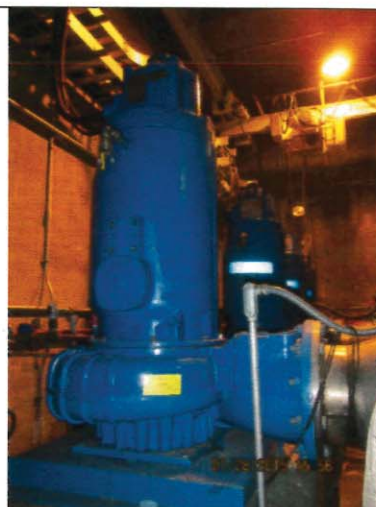
Photo 12: MAPS dry well pumps
