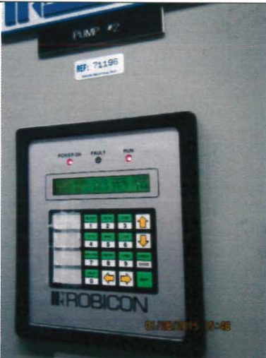
Photo 11: MAPS variable frequency drive for Pump #2 (lead pump)
