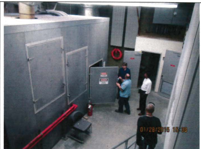
Photo 6: MAPS main floor with enclosed diesel generator
