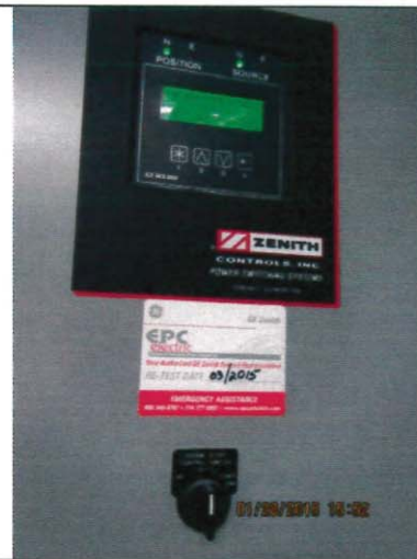
Photo 8: MAPS automatic power transfer switch and service testing sticker with re-test date indicated as 03/2015.
