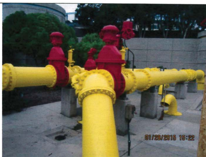
Photo 2: Moss Avenue Pump Station (MAPS) compound and dual force mains
