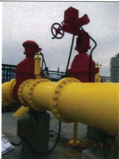
Photo 3: MAPS force main air relief valves and motor-actuated bypass valve
